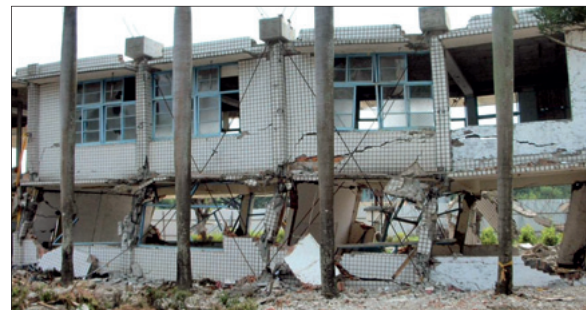
Fig.1 In-situ tests (in collaboration with USA and Mexico) of school buildings at Guan-Miao Elementary School in Tainan
