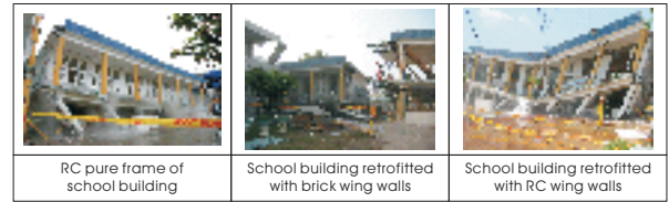
Figure 3-1 School building seismic ability on-spot inspection at Ko-hu Elementary School of Yunlin County
